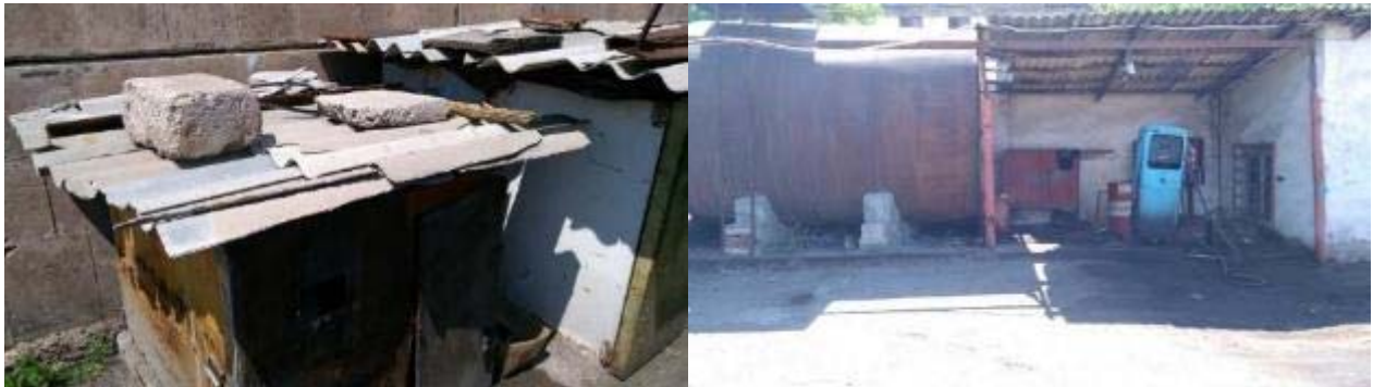
Figure 4-13. Roof elements containing ACM in Nor Nork (Jrvej) and Charbakh bus depots
