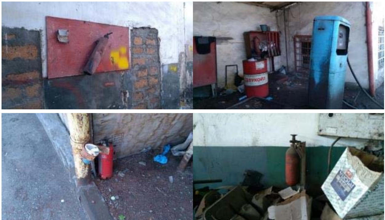
Figure 4-22. Primary fire-fighting equipment unsuitable for use at Charbakh depot
