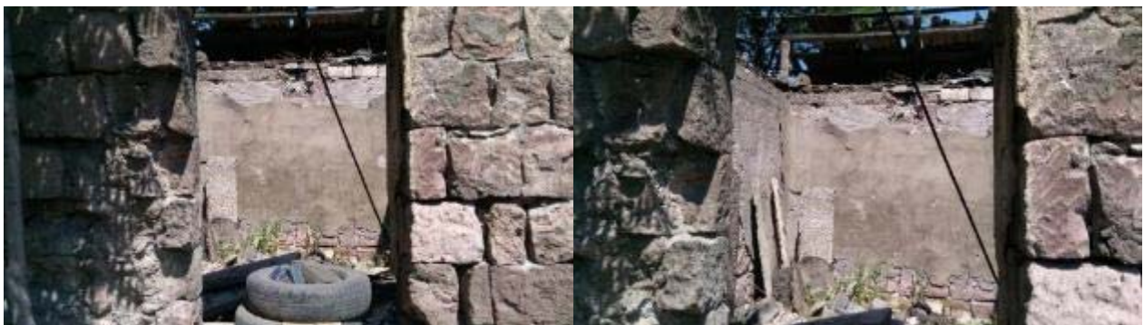
Figure 4-4. Damaged and largely demolished building in Charbakh depot
