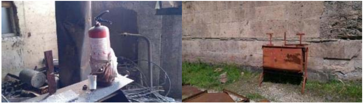
Figure 4-21. Primary fire-fighting equipment unsuitable for use at Nor Nork (Jrvej) depot
